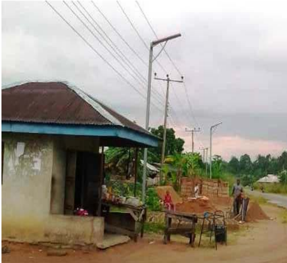
FUNCTIONING SOLAR STREET LIGHT AT OBOHIA, UKWA EAST LGA, ABIA STATE
