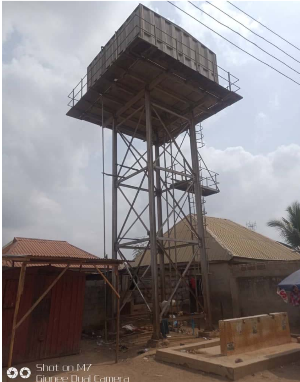
NON-FUNCTIONAL BOREHOLE, KAGINI, BWARI AREA COUNCIL
